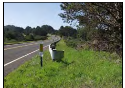
Guardrail on Highway One, between Brewery Gulch and Chapman Pt Rd.
