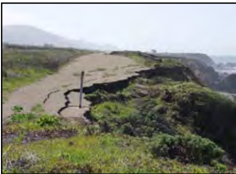
Road washouts, old Coast Highway, Westport-Union Landing State Park
